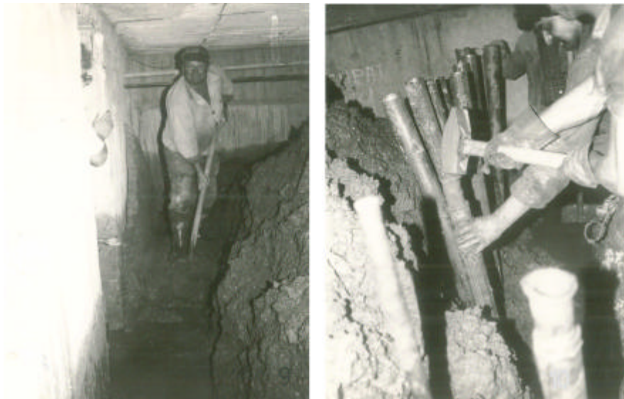
Figure 5. Creating the working place and introduction in soil of the pipes that constitute the stopping screens
