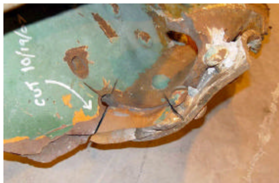
Figure 3. Gusset Plate fractured
