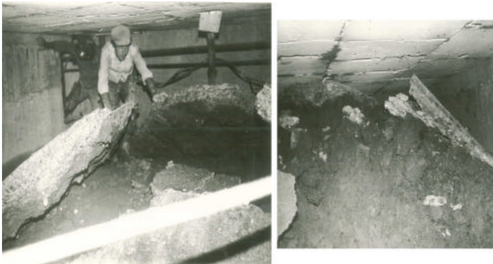
Figure 2. Displacement and shifting of floor from the basement
