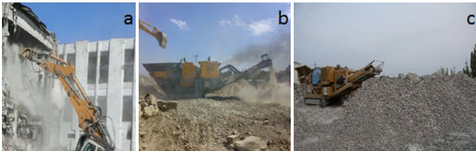
Figure 1. Typical demolition site of a building: a – demolition of the cement concrete structure of the construction; b – crushing of the demolished cement concrete; c – storage of the obtained recycled aggregates
